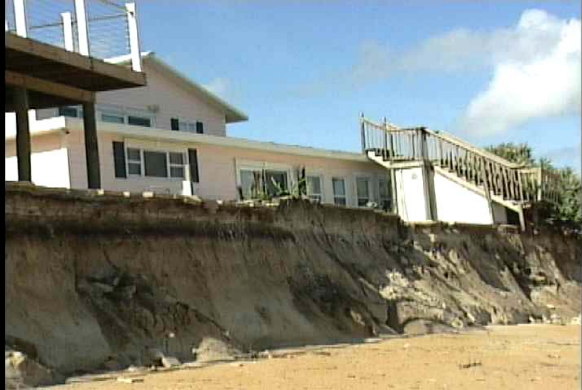
© 2010, Central Florida News 13, LLC. All Rights Reserved - http://www.cfnews13.com/News/Local/2007/12/23/severe_erosion_damages_several_homes.html
