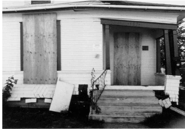
Figure 10 - This home wasn't bolted and slid off its foundation. Sometimes the damage can be so bad that houses have to be demolished.
