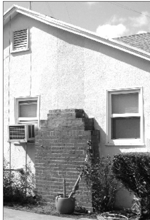
Figure 31 - Photo showing damaged chimney removed. Note that the fireplace is now not functional.
