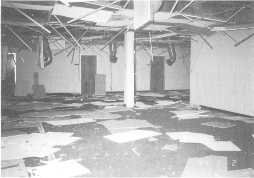
Earthquake Damage: 1994, Northridge, California Photo Credit: Wiss, Janney, Elstner Associates, Inc.
