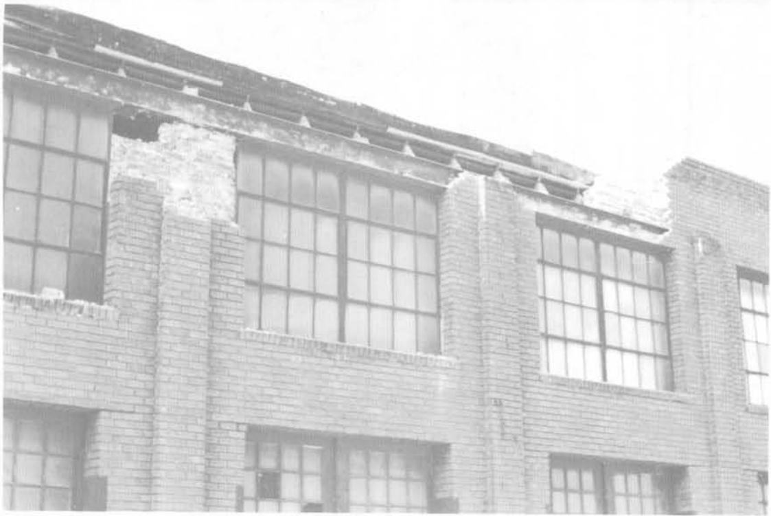
Earthquake Damage: 1989, Loma Prieta, California Photo Credit: Wiss, Janney, Elstner Associates, Inc.
