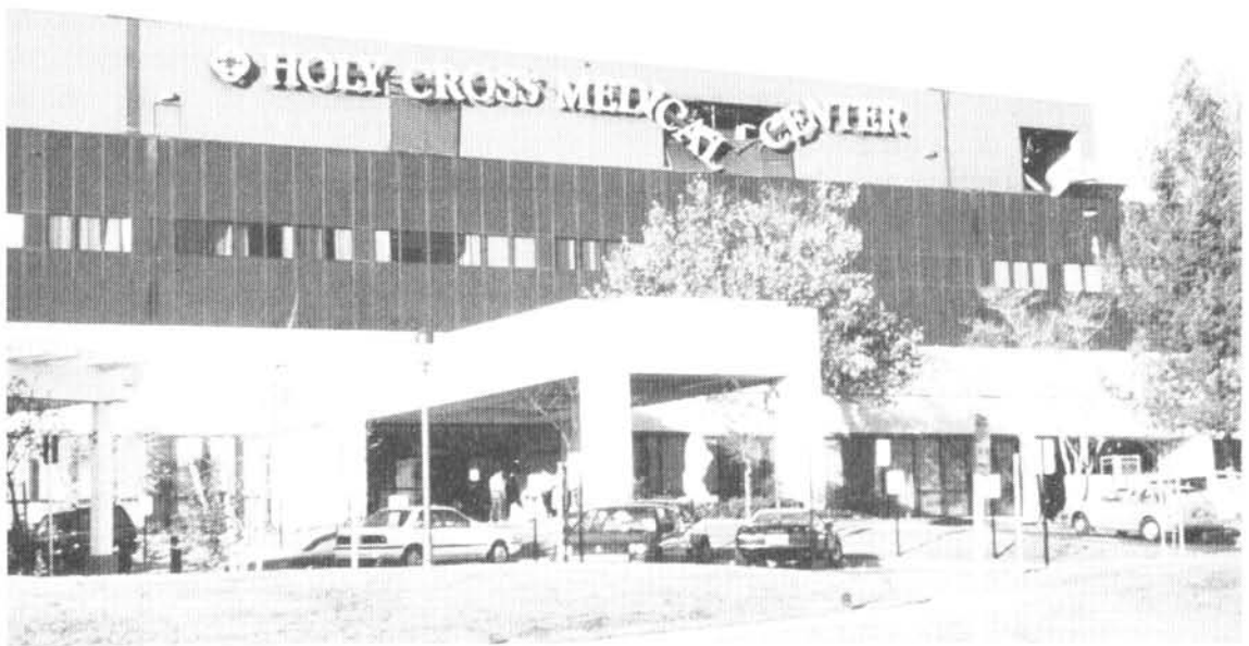
HVAC damage at Holy Cross Medical Center in Sylmar—damage to signage and louvers caused when suspended fans in the mechanical penthouse swung and impacted the louver panels. HVAC service outage caused the temporary evacuation of all patients. Earthquake Damage: 1994, Northridge, California Photo Credit: Robert Reitherman
