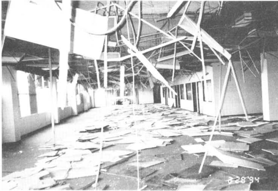
Complete loss of suspended ceiling and light fixtures Earthquake Damage: 1994, Northridge, California Photo Credit: Wiss, Janney, Elstner Associates, Inc.
