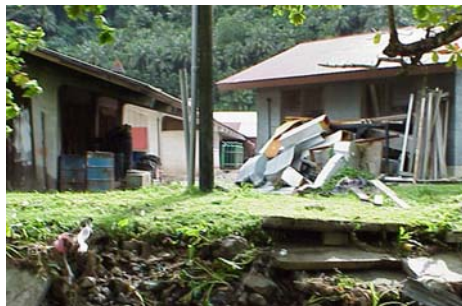
Flood damage included the island's only hospital, LBJ Hospital, during a May 2003 storm.
