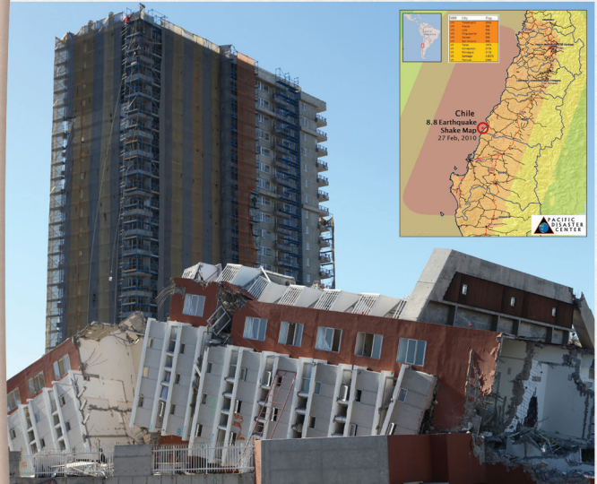
Experts believe the risk of another large earthquake in Chile, an APEC member economy, remains high. This image shows a high-rise apartment building in Concepcion that collapsed as a result of a magnitude-8.8 earthquake that struck on February 27, 2010. Inset: USGS Shake Map. (Image courtesy of the U.S. Geological Survey, Walter D. Mooney, Photographer)
