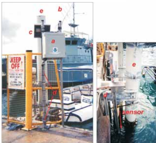
Rarotonga sea level station, Avarua Harbor, Cook Islands. The fiberglass electronics package (a), antenna (b), solar panel (c) were installed on a pier. Conduit (d) containing cables connecting the sensor, located at a depth of five feet below low-tide water level, to the data collection platform containing the electronics above, was externally attached to the tube containing the sensor (e).
